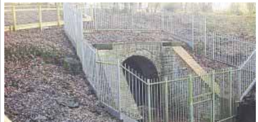
Restored northern portal of the Tyler Hill Tunnel on the University of Kent campus
